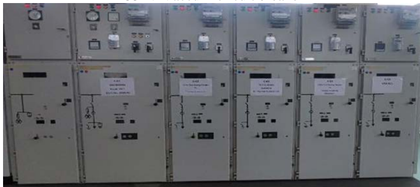
12 kV Vaccum-circuit breaker Switchgear
